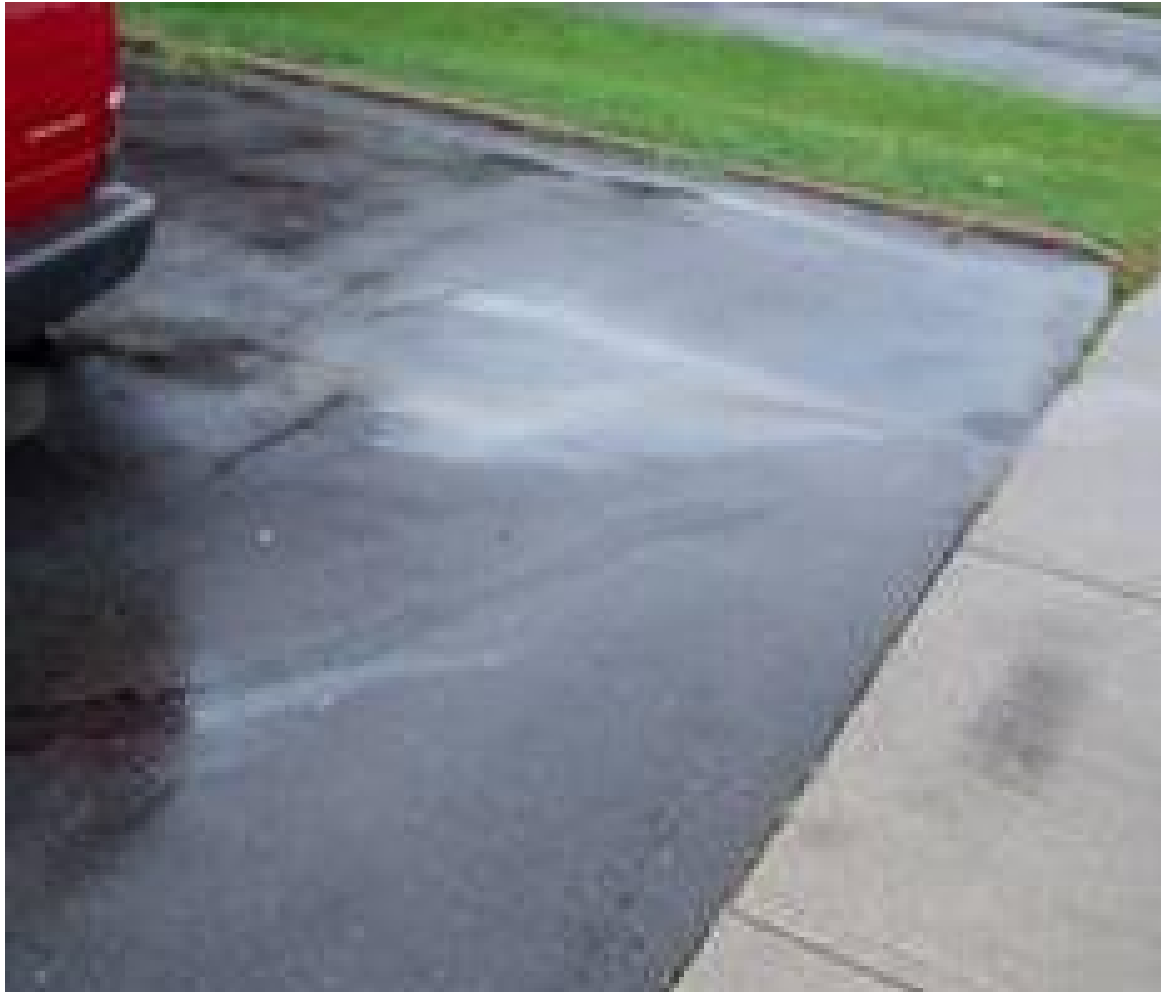
Oil runoff from impervious parking pavement
