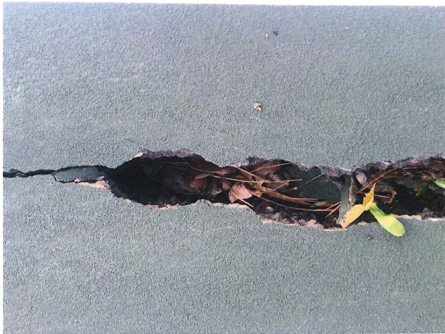
Photo 2 - Debris Accumulation in Crack
