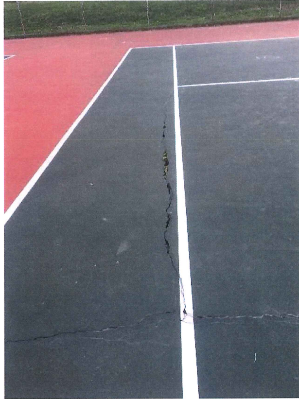
Photo 1 - Debris Accumulation in Crack
