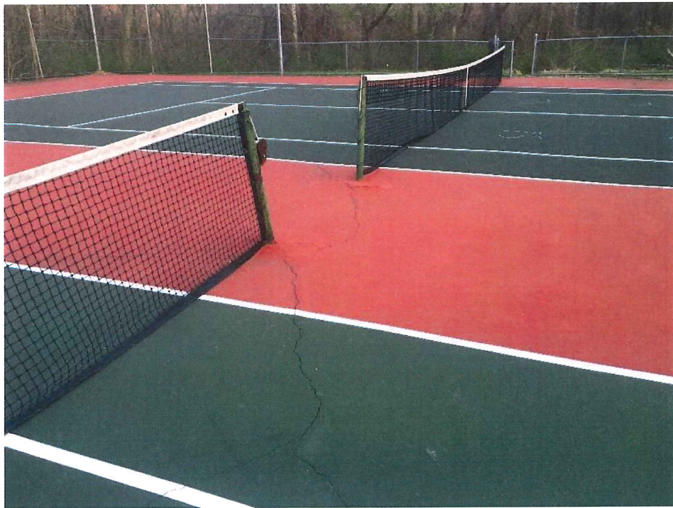
Photo 4 - Crack Beginning at Net Post
