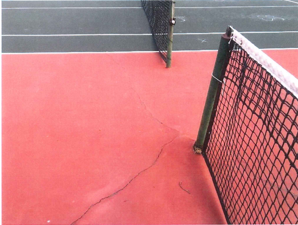
Photo 5 - Crack Beginning at Net Post
