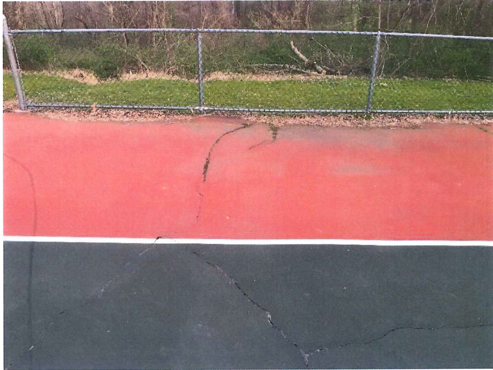
Photo 3 - Vegetation Accumulation in Cracks
