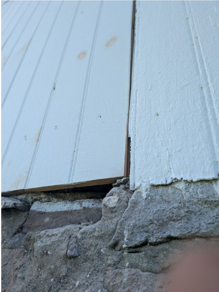
Photo 1 – North Side of Patterson Main Barn – Unprimed cuts on edges and bottom, wood used was not adequately prepared or clean lumber(bleed through of sap), highly likely that coating does not meet required thickness. Note that multiple wood patches at both main barns on multiple elevations exhibit this flash through. Fastener issue noted in previous
