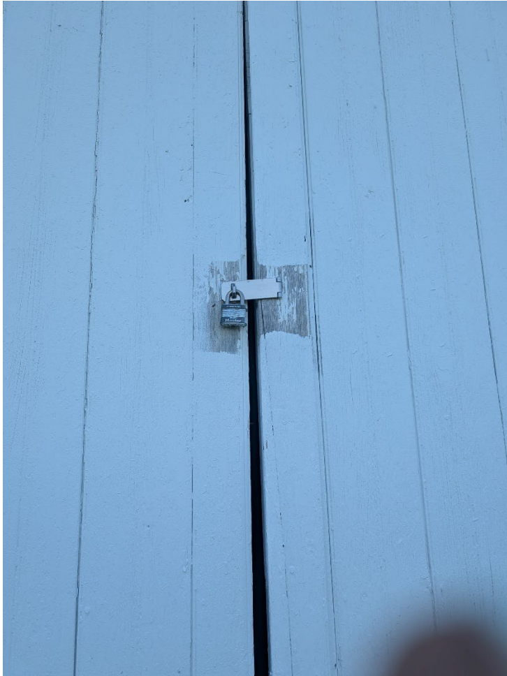
Photo 6 Patterson Main Barn West Side. Note area not painted. Spray pattern on left indicates possible mil thickness issue where paint was applied.
