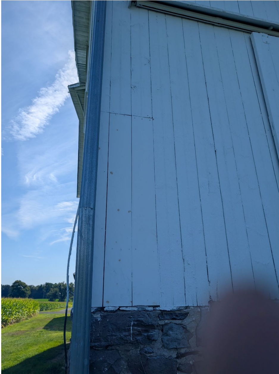
Photo 2 West Elevation of Patterson Main Barn. No profile on wood patch, wood has bleed through with sap, fastener type not corrected from previous report, likely paint drip from this work. Note all patches were square cut at the horizontal cuts rather than beveled which is the preferred cut to shed water.
