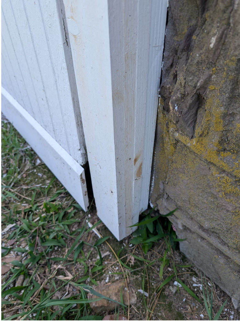
Photo 7 Door Repair at Patterson Main Barn. Unpaint cuts, new lumber insufficiently painted, questionable strategy for protecting bottom edge of door and certainly not 'historic'
